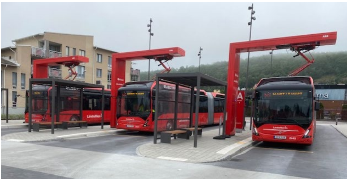
Figure 6. Buses charging by pantograph at the end station in Jönköping
